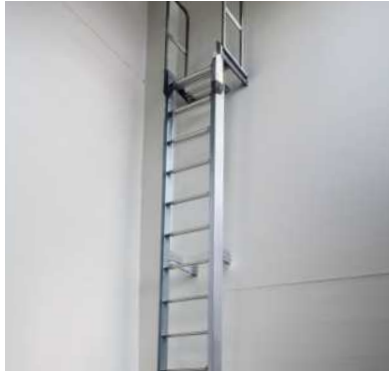
Wall-Mounted Industrial Ladder
